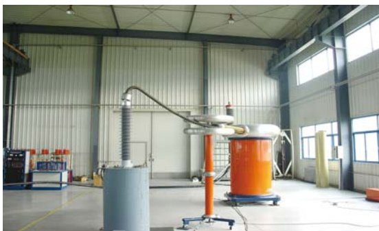
Testing Transformer Bushing
