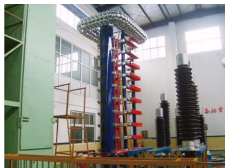
High Voltage Test Equipment
