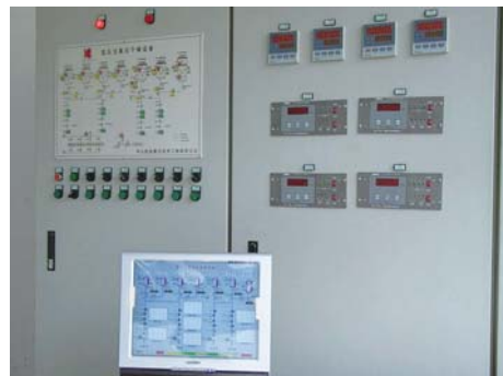
Vacuum Drying System for condenser core
