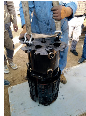
Figure 7: Resistive Type OLTC as removed for inspection
