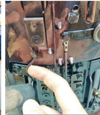
Figure 8: Broken contact for the wire connecting the transition resistors to the transition arcing contact in Phase B
